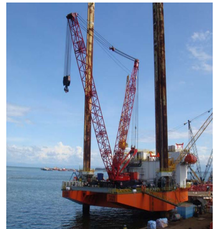
2007- 1200 te capacity crane mounted on the Global Process System Sdn Bhd jack up barge in Malaysia.
