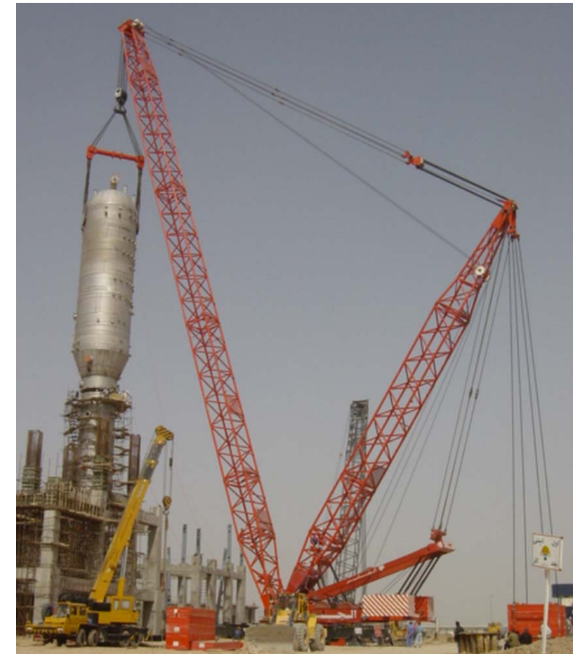
Erecting a 360 te demethanizer in Iran at 30m above ground level in Iran.
