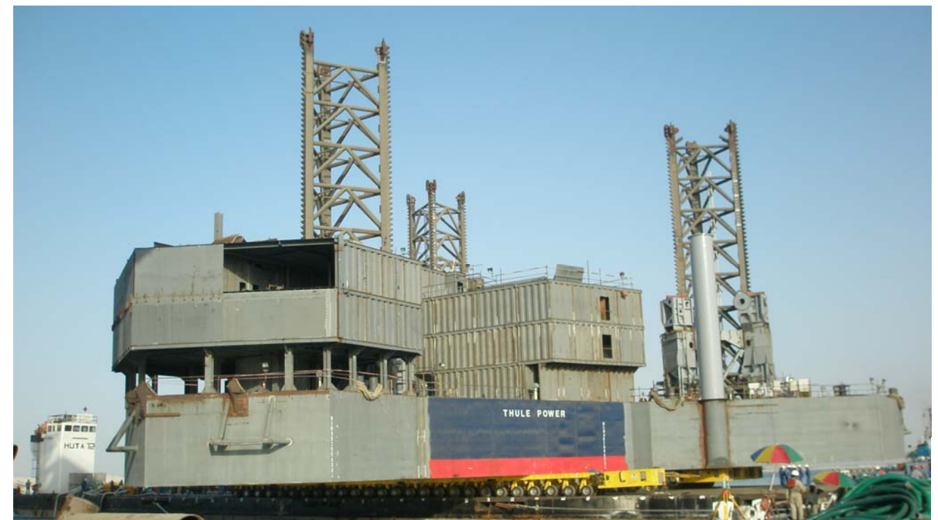
Weighing a 4015 te of rig hull "Thule Power" by means of 154 SPMT Hydraulic axle Lines and marine load out onto barge in the U.A.E
