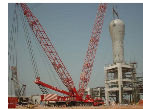
Erecting 400 te reactor into a 17m high structure Using a Gottwald AK 912 in U.A.E
